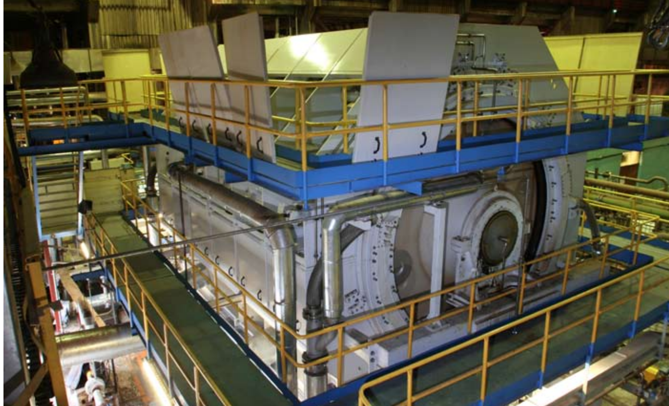
As part of the fiberline upgrade, SPPM replaced its old washing system with a two-stage DD Washer.
