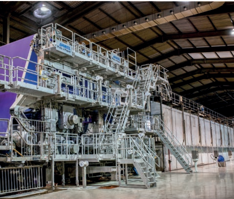
▲ ANDRITZ installed a new press section on Iggesund’s BM2, including a long-nip jumbo press with large-diameter rolls, an energy-efficient PrimePress X shoe press in the second nip, and a smoothing press. The delivery also included ANDRITZ’s state-of-the-art PrimeFeeder vacuum system for ropeless tail threading from the press section to dryer section.
