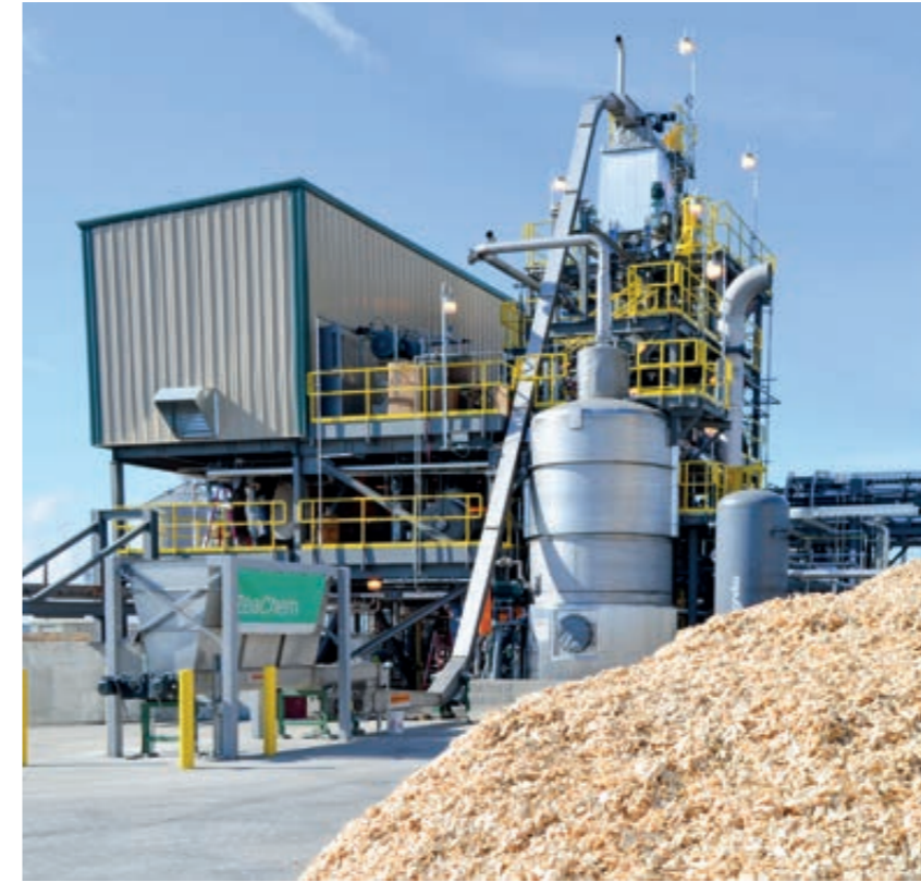
◀ Pretreatment and hydrolysis equipment at Boardman
