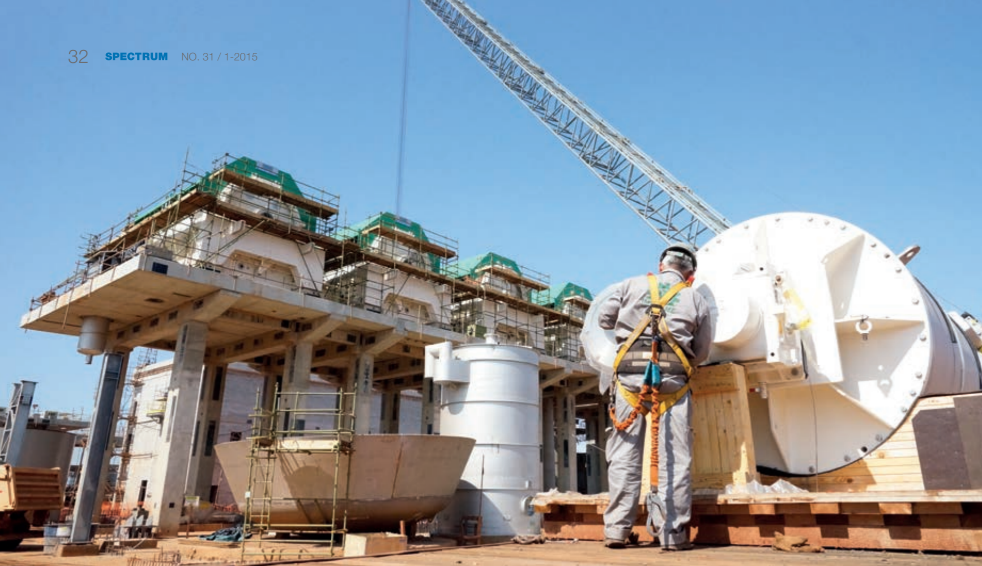
◀ Annual production capacity will be 1.5 million tonnes (1.1 million tonnes of hardwood and 400,000 tonnes of softwood). A sizable portion of the softwood will be produced as fluff pulp. Shown here is the ANDRITZ fiberline under construction.
