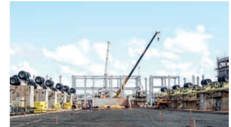
The ANDRITZ woodyard will have four debarking drums (structure for two of them shown in the foreground) four chippers, and two massive 360-degree stacker/reclaimers. ▼
