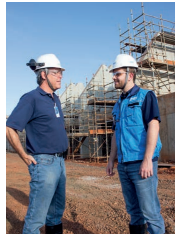
◀ ANDRITZ'S Bruno Salamone, Project Engineer (left), and Olavo Filipecki, Project Manager, look over construction progress in the woodyard.
