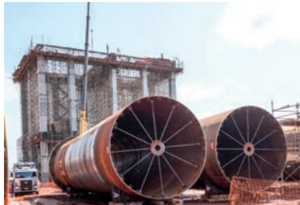
There will be two kilns in the white liquor plant (650 t/d each). The building in the background will house equipment for green liquor filtration and white liquor preparation. ▼
