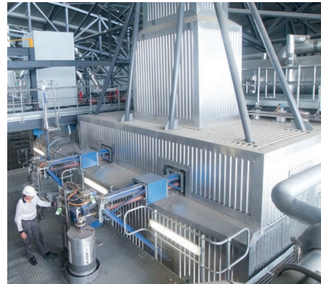
▲ The EcoFluid boilers are being commissioned and started up on a staggered schedule. The Tuen Mun facility is currently operating with two boilers and a throughput of about 660 t/d of sludge. Shown here is Johannes Geiger, ANDRITZ Commissioning Manager, checking the instrumentation at one of the boilers.
