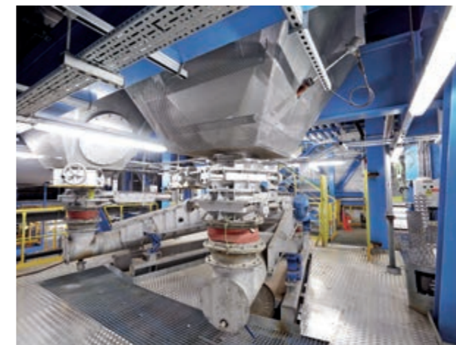
▲ Vibrating bed-ash dischargers of 1 st pass before particle separation.
