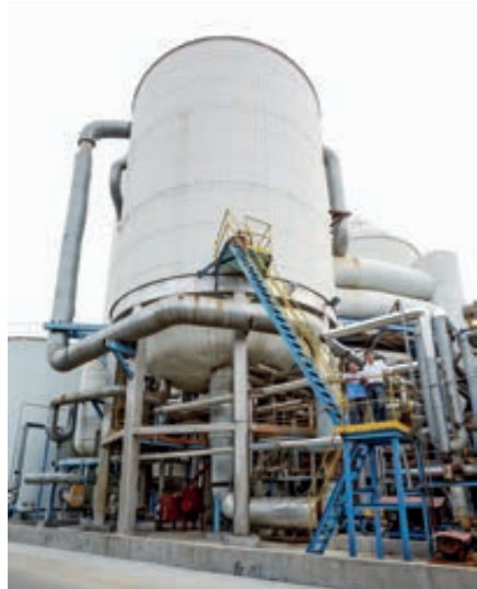
▲ Zedivap effluent evaporation unit for zero effluent from the mechanical pulping line
