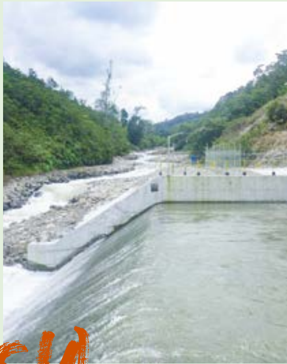
Hasang, North Sumatra, 3 × 13.73 MW
