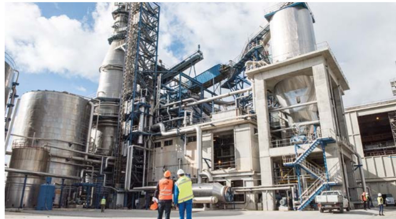
ANDRITZ supplied the latest technology for the digester and chip feeding system at Celbi.
