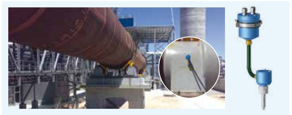
▲ The location of the ACU-230 sensor installed on a lime kiln carrying roller friction bearing. The sensor features a separate sensor head and electronics in separate aluminium enclosure, ideal for applications with high temperature at the monitoring area.
